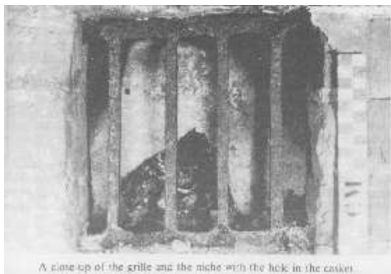
A close-up of the grille and the niche with the hole in the casing.
